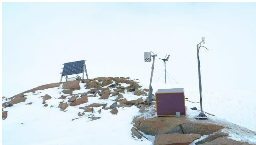
Figure 2: View of the installation at the CLIMB remote
